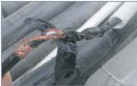
Wiring Fault Case
